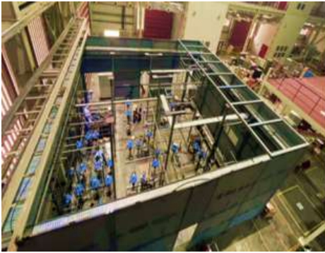
Figure A.4.12: Bird's eye view of the EHCL system at site.
