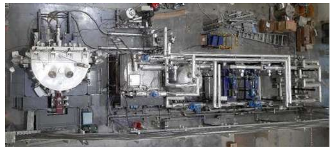
Figure A.4.9: A bird's eye view of the high heat flux test facility in operation.
