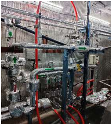
Figure A.4.33: Cooling water system of TS.
